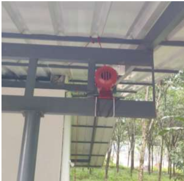
Figure 4: Photograph of Alarm
